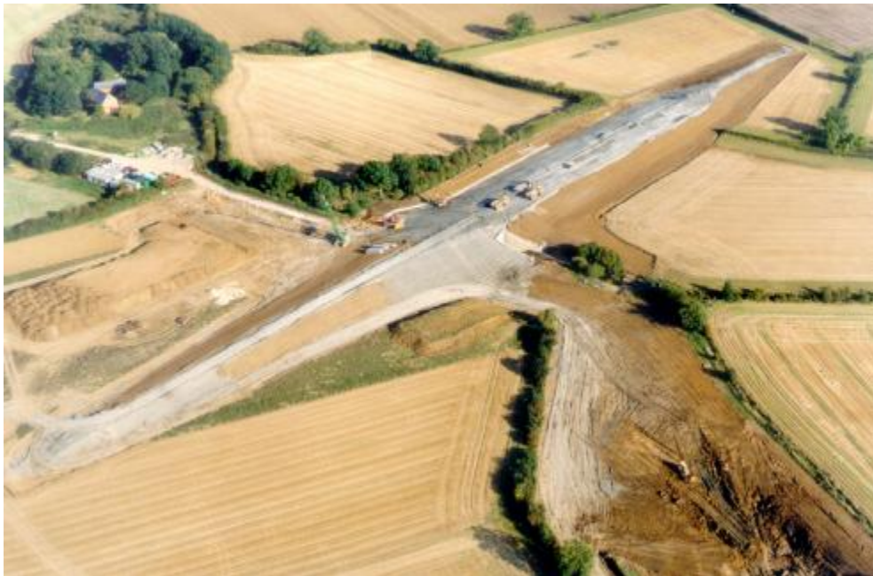
Figure 1. Weedon Dam under construction. The borrow pit is at the lower right. Note retained tree and hedge lines screening the embankment.
