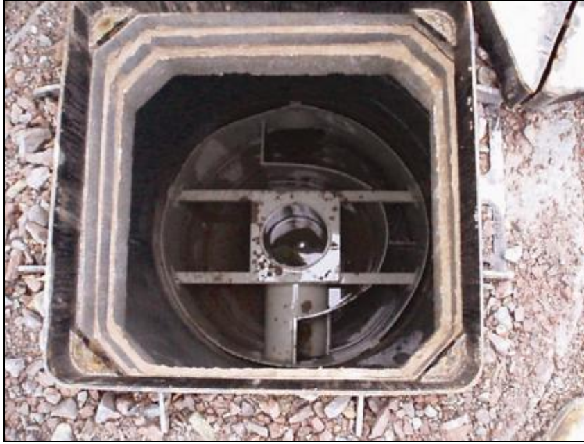
Figure 6. Downstream Defender® hydrodynamic separator – silt and sediment removal device used prior to infiltration devices and ponds
