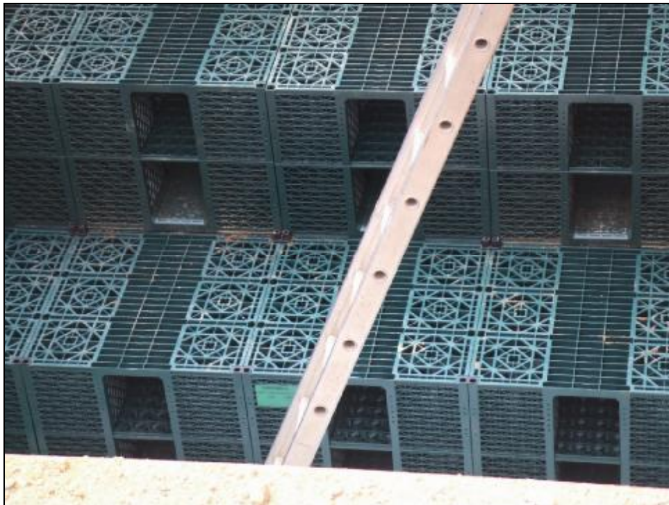
Figure 5. Stormbloc® geocellular modules during the construction of one of the infiltration trenches at Lightmoor
